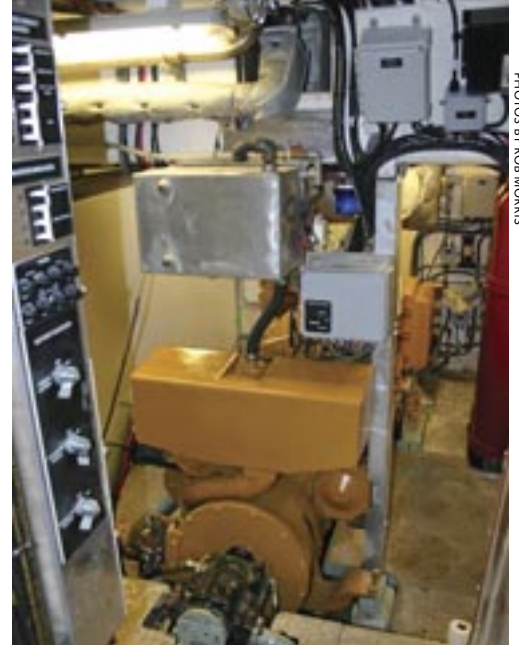
The 275-hp Caterpillar 3406 main on Twin Disc 5114 (3.5:1) marine gear provide 10.5 knots top speed at 1850 rpm. At nine knots (1500 rpm) fuel consumption is approximately five Imp. gals/hour. Fuel capacity is approximately 1450 Imp. gals. There is a 9 kW Kubota genset.
